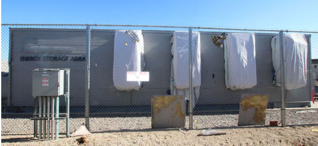
Figure 4.5: Photograph of the ESS after the incident from the northwest [13].
