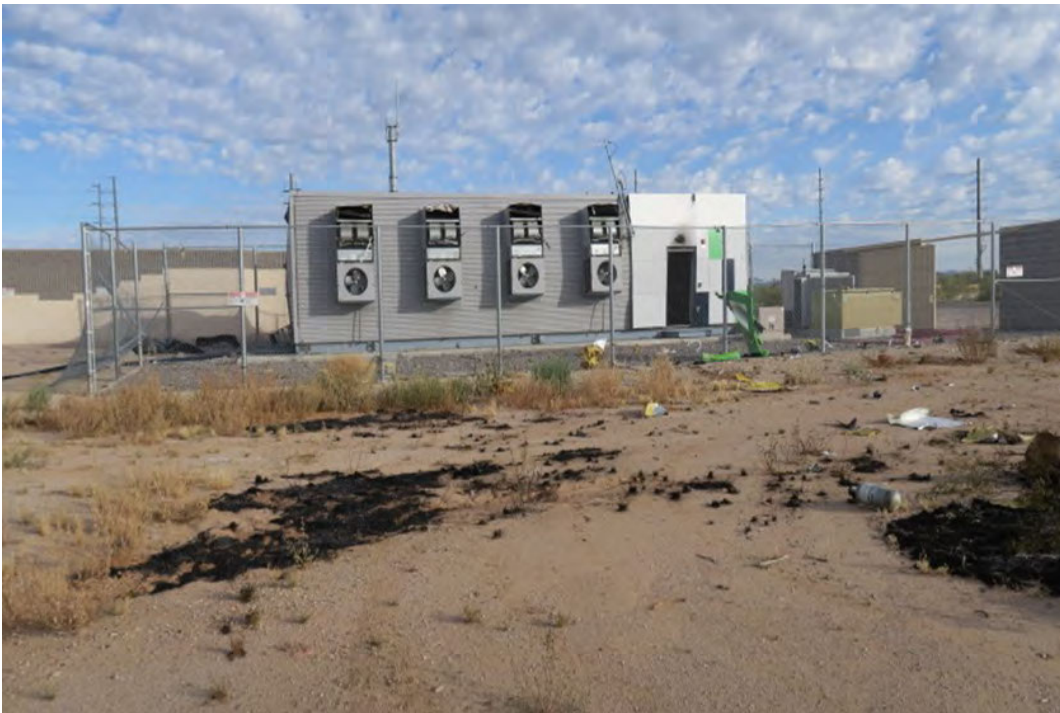
Figure 4.20: Photograph of fire debris and SCBA tank removed during the deflagration [6].
