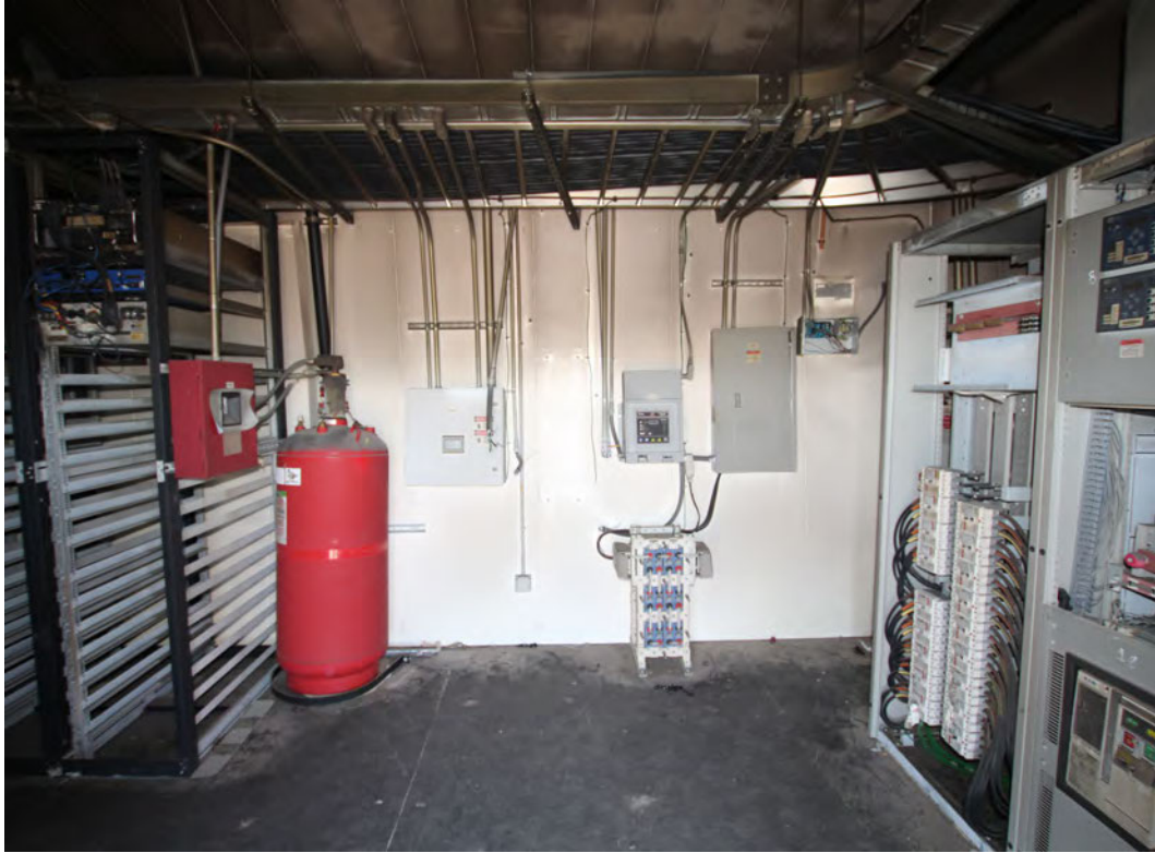
Figure 4.15: Photograph of view into the ESS from the entry door [13].
