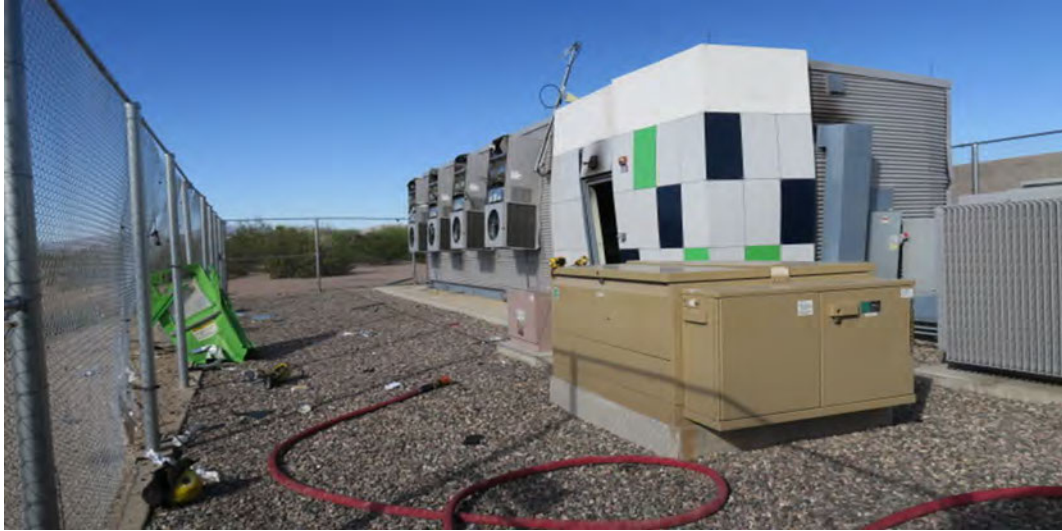
Figure 4.18: Photograph of firefighter helmets and the door to ESS removed during the deflagration [6].
